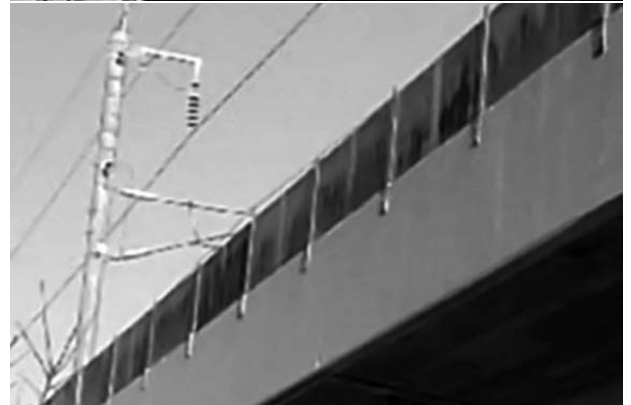
Peeling and flaking on concrete viaduct (top) After repair work (bottom) (JR East)
