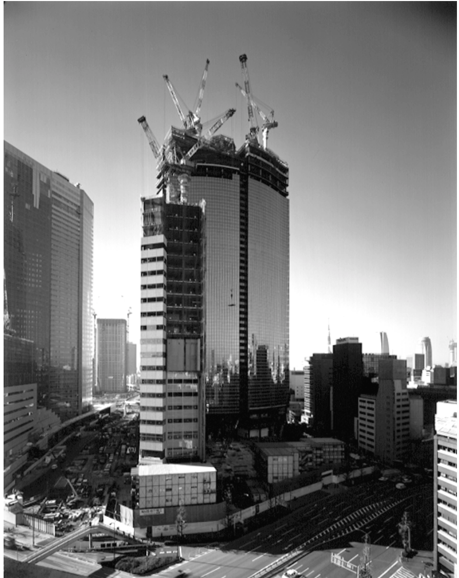
High-rise office and residential buildings under construction on the former site of Shiodome Freight Terminal. Restoration of the old Shimbashi Station at the north end of the site is scheduled to be completed in spring 2003 to commemorate the birthplace of railways in Japan. (Mitsui Fudosan Co., Ltd.)
