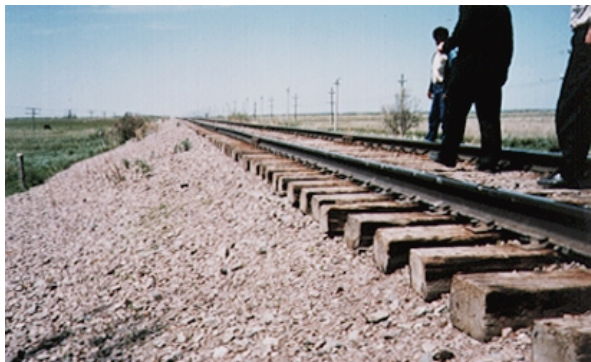
The ballast on this single track in Eastern Kazakhstan which runs from Aktogay to Druzhba (and further east to China) has been left unattended for 30 years.
