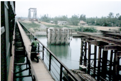
Building a new railway bridge alongside a damaged existing bridge to increase track speed and capacity.
